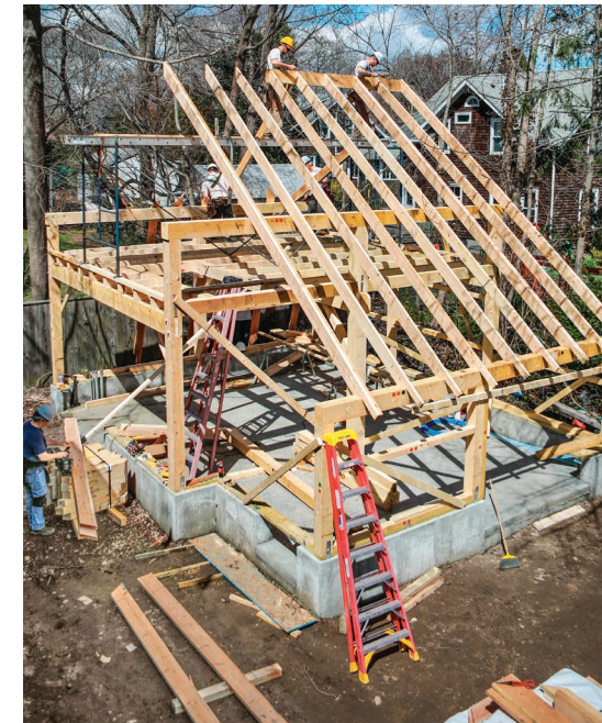
RIGHT: The post-and-beam barn arrived on-site in kit form. Cutting the barn frame at a factory, rather than on-site, saved time and money. After assembling the frame, the crew cut, then installed, the 2x12 rafters.
